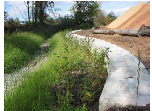
Realignment After 2 Months
